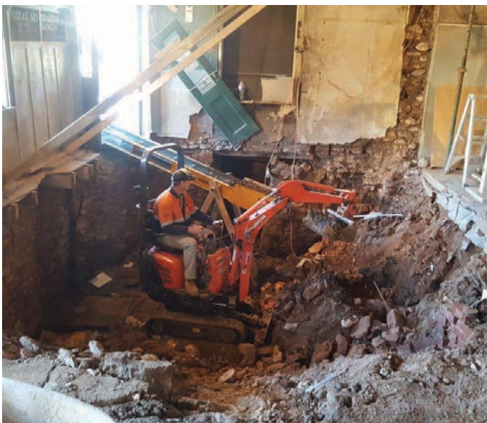
John commented that the local tradesmen had been fantastic throughout the renovation period, and could not have asked for a better group of workers – no job was to great or too small – they
